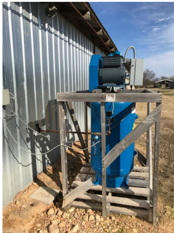
Figure 22. FBCS compressor with vertical air reservoir configuration as installed at poultry house
